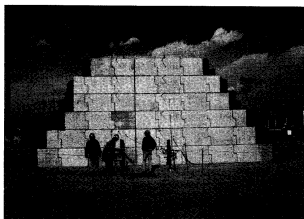
Photo 7. Concrete block front-face stretch-made polymer grid (SR) reinforced retaining wall (for testing in 1986)
